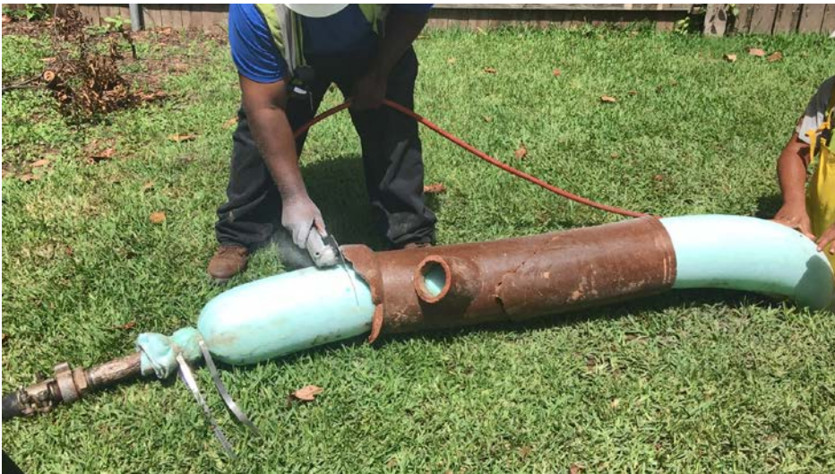
Figure A8. Employee cutting excess section of steam-cured liner outside of manhole at CIPP installation, June 2019. Photo by NIOSH.
