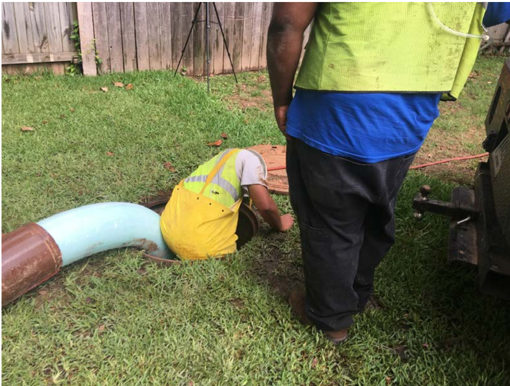
Figure A7. Employee cutting steam-cured liner partially inside of manhole at CIPP installation, June 2019. Photo by NIOSH.
