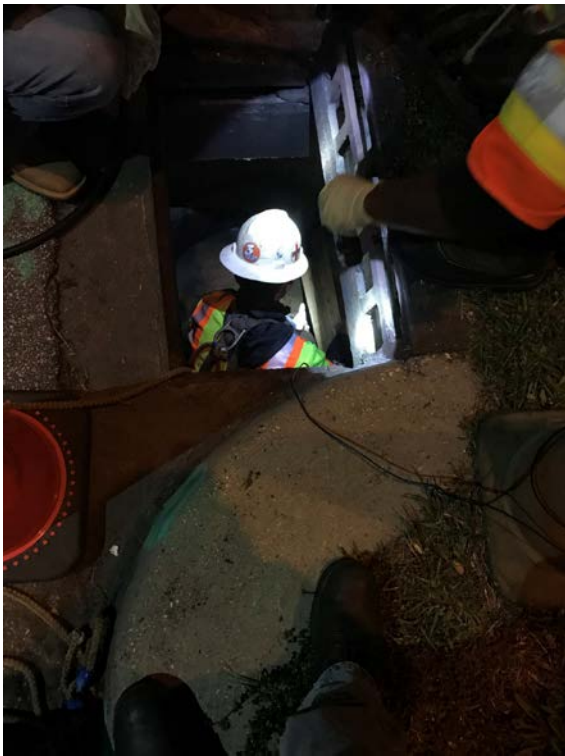
Figure A6. Employee cutting water-cured liner inside of access hole at CIPP installation, March 2019. Photo by NIOSH.
