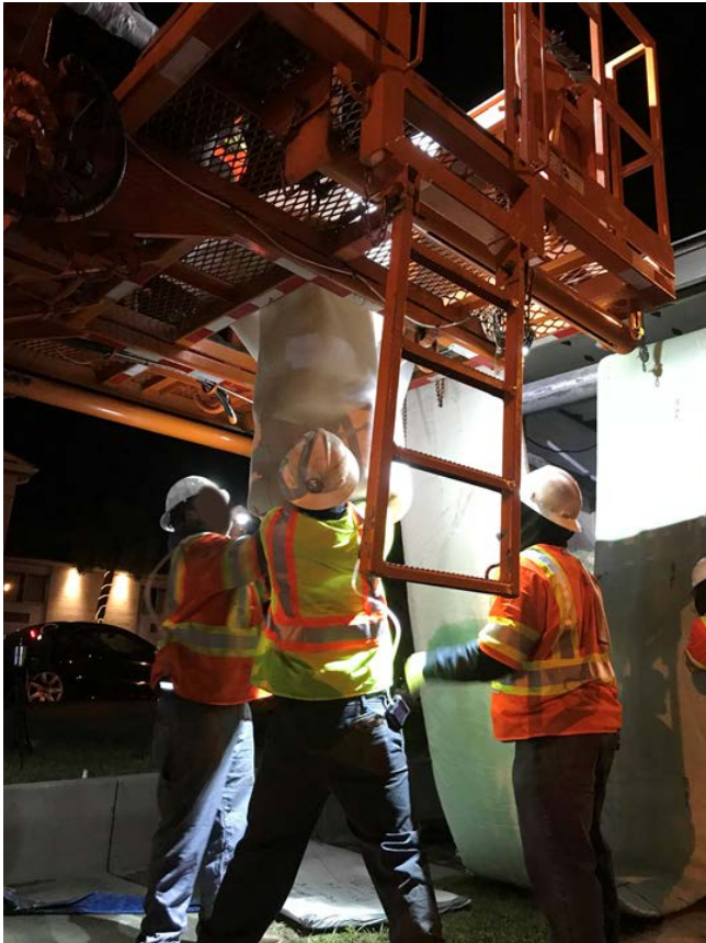
Figure A5. Employees pulling dry liner through itself under lift on boiler truck during water-cured CIPP installation, March 2019. Photo by NIOSH.
