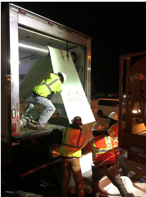
Figure A4. Employees removing liner from refrigerated truck during water-cured CIPP installation, March 2019. Photo by NIOSH.
