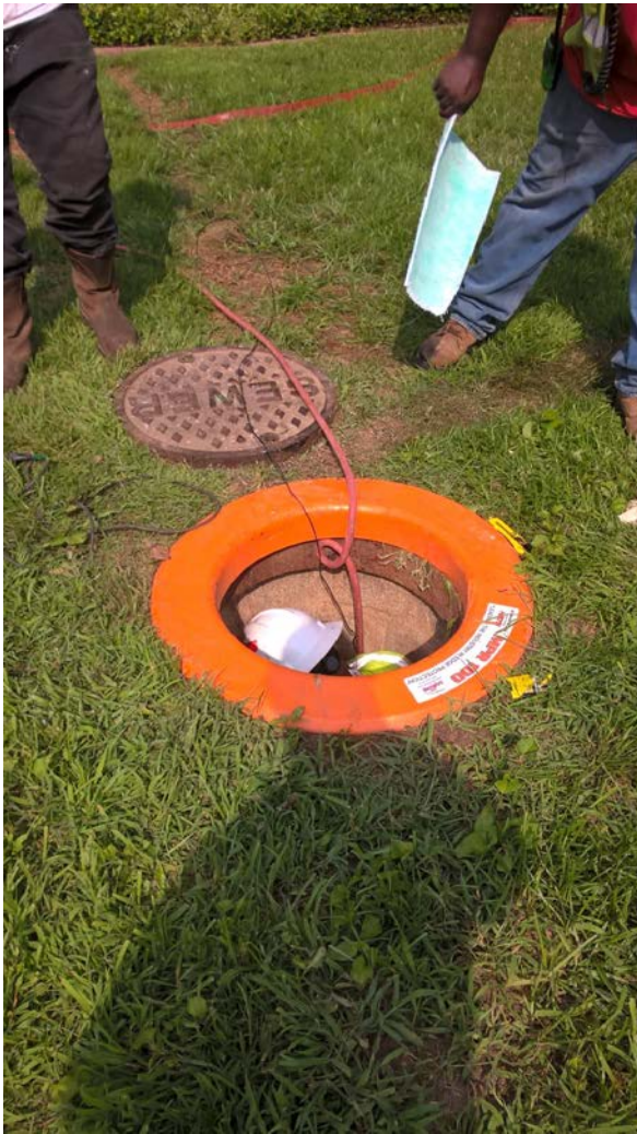
Figure A9. Employee cutting steam-cured liner fully inside of manhole at CIPP installation, June 2019. Photo by NIOSH.
